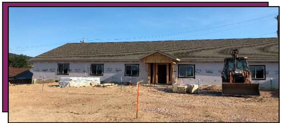
Wright Street during the construction process, photo courtesy of Black Hills Works.
