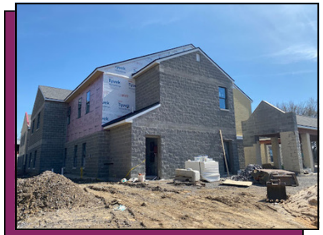
Dogwood Springs, under construction, photo courtesy of the Helen Ross McNabb Foundation
